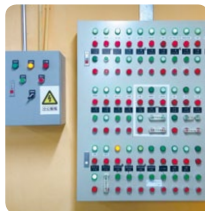
Small zone lighting system
