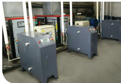
Energy recycling system
